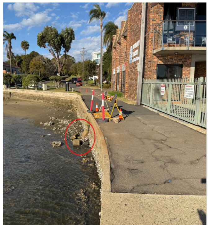
Figure 2: Failure of sandstone seawall
