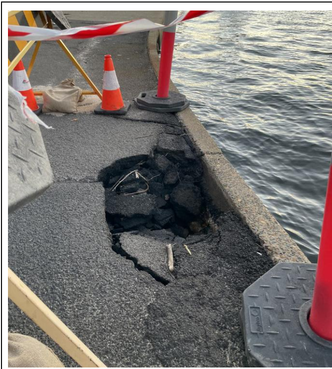
Figure 1: Failure of the asphalt accessway
